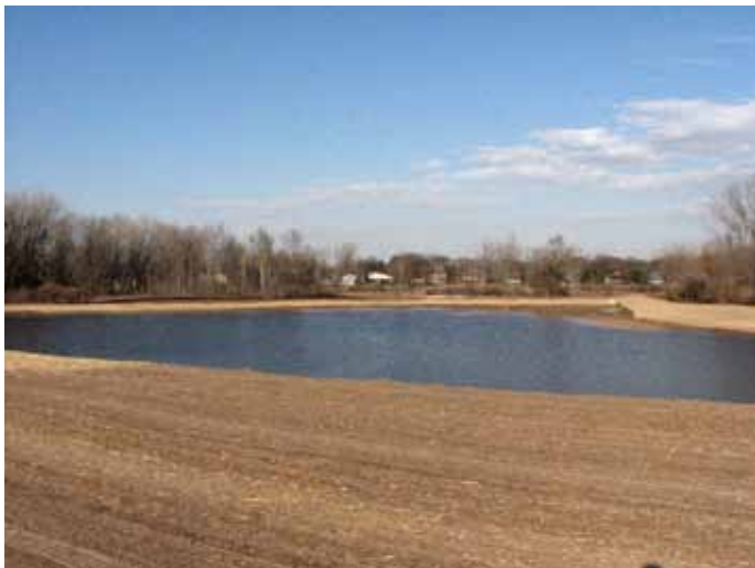
Restoration work at the Wheeler Rd. ponds will continue through the winter. Photo by Jan Axelson.
