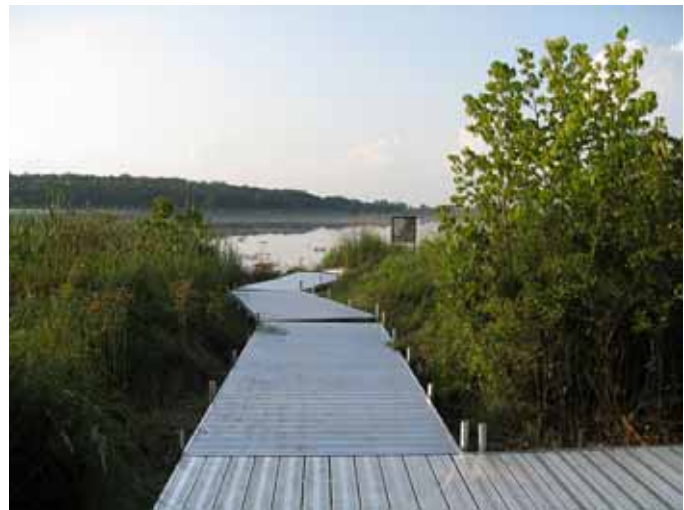
The new boardwalk (shown here under construction) has wide teaching platforms for school groups. Photo by Jan Axelson.
